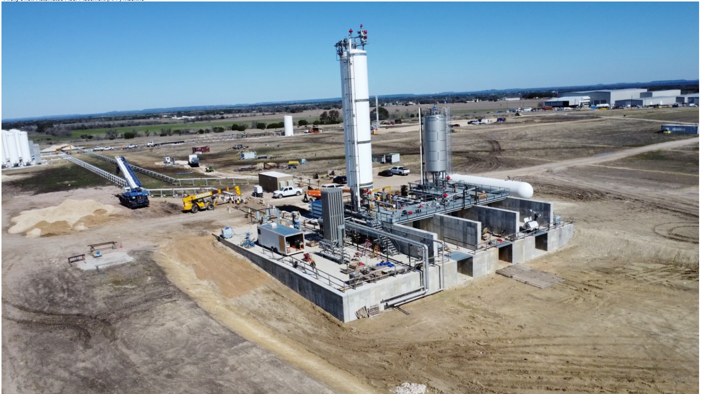
*Firefly's new multi-bay engine test stand for MLV's first stage Miranda engines and second stage Vira engine
